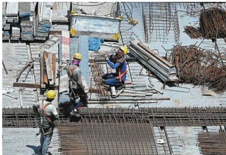
One expert suggested the construction industry change its practices so that workers start work earlier in the day and have a break in the afternoon, during the hottest times of the year. According to the Workplace Safety and Health Guidelines, heavy physical labour or work under the sun should be done during the cooler hours of the day. ST PHOTO: DESMOND WEE
